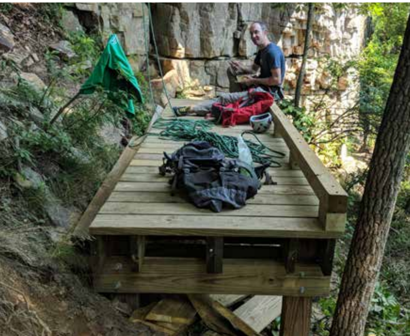
A newly constructed belay platform above a watercourse at Denny Cove gives climbers a safe and dry place to belay and protects the surrounding ecosystem from erosion and rapid degradation.
